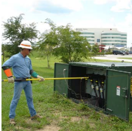
A 3-phase SF6 switch used in electrical utility distribution.
